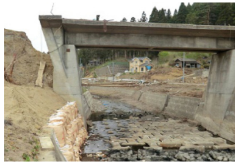
Fig. 7: Seaside view at Yonedagawa bridge in Noda village after tsunami affect, Iwate prefecture
