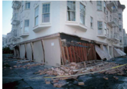
Fig. 5 Apt. Building - Loma Prieta, CA, EQ – 1989 (Soft story)
