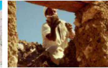
Fig (8.2): The walls are built using kershef natural material to keep the rooms cool
