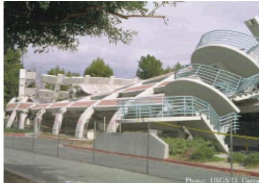
Fig. 4 Parking garage – Northridge, CA, EQ – 1994 (Inadequate capacity of non participating elements)
