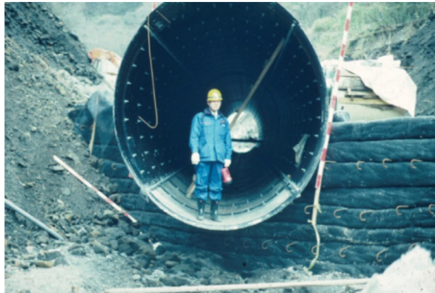
Fig. 3: Reconstruction works of railway embankment failure in Kyushu in 1991 by GRS RW technology [8]
