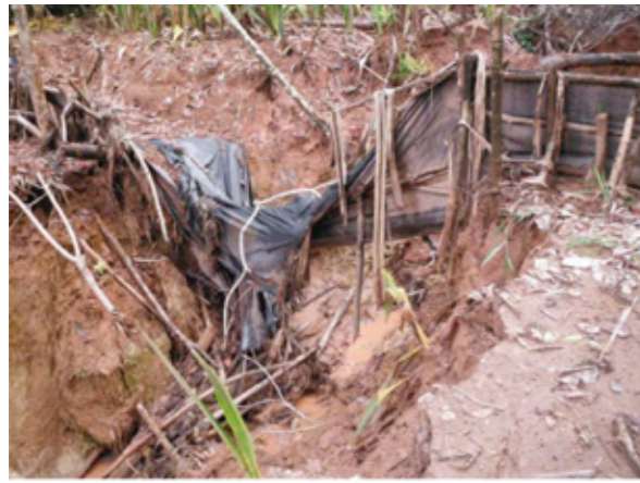
Fig.11 The outflow of the stored red clay
