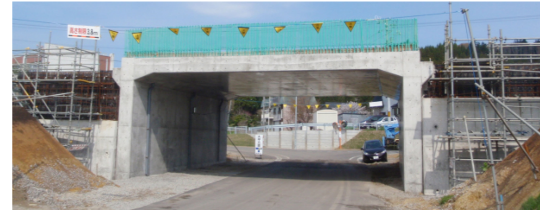
Fig. 13: First GRS integral bridge for a new high-speed train line at the south of Hokkaido: a) structural details (the width= 11.7 m); b) during construction (August 2011); and c) nearly completed (August 2012).
