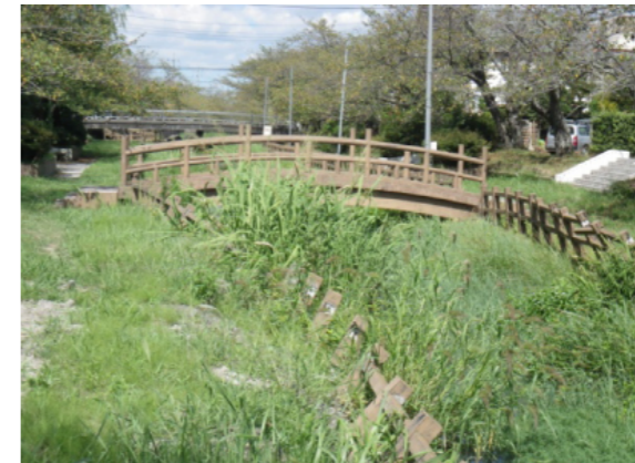
Fig. 6: Lateral flow of level ground facing at chanel in Katori city, Chiba prefecture
