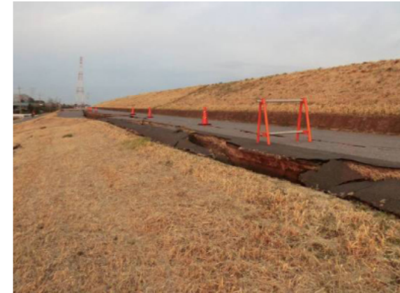
Fig. 5: Cracks on Tone river levee, Kitasoma district, Ibaraki prefecture
