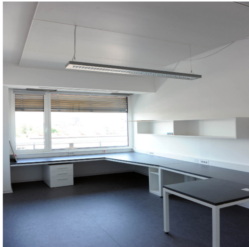
Illustration 3. The heating/cooling ceiling panels in refurbished offices.
