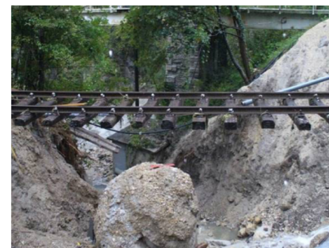
Fig. 2: Railway embankment that failed by rainfall and flood in September 2010 in Zagorje, Slovenia
